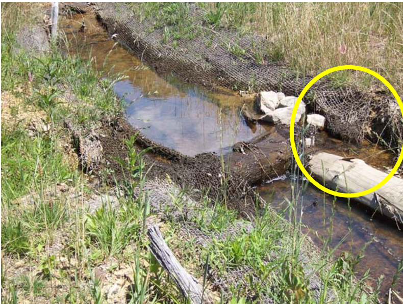
Figure 7. Erosion at Vane 30 June 2007 (yellow circle).
